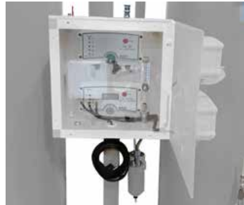
BM sensing panel (includes O 2 , CO, CO 2 monitoring)
